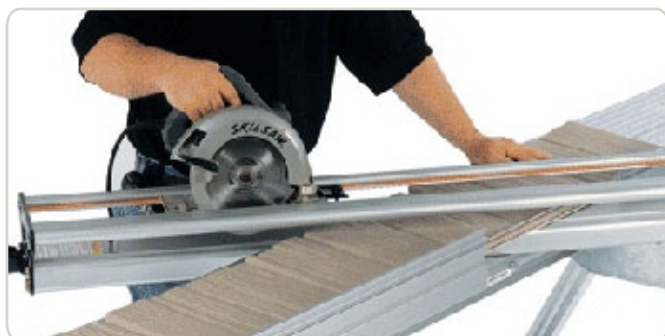
Fig. 21. For cutting thin metal on site, we recommend a circular saw with metal cutting blade
